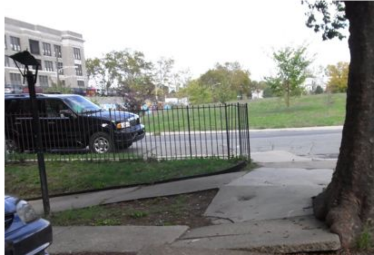
SIDEWALK CONDITIONS Tree breaking through the sidewalk pavement. Along Haverford Avenue, there are signs of street trees being removed.
