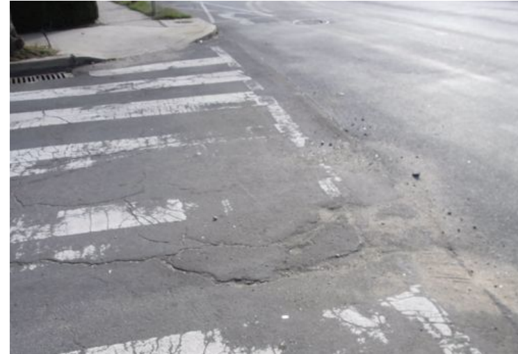
SUBSIDENCE Historically, subsidence has been an issue
